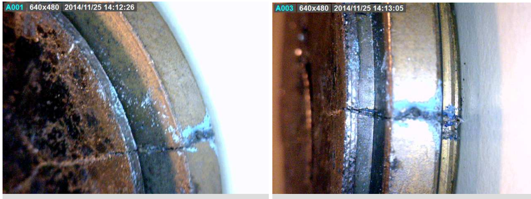
Figure 14 ESFR-363 Button – Images of Post-Stress Corrosion Cracking of Brass Parts Test
